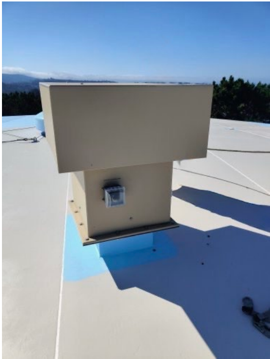
West Belmont (N) –Blower installed
